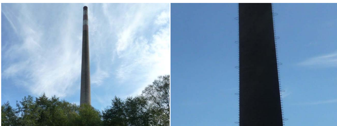
Figure 12 – View of the chimney from the northwest and detail of the metal ladders
